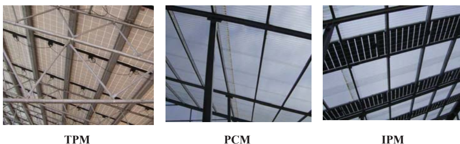
Fig. 1. Details of greenhouse cover material: (TPM) traditional photovoltaic modules; (PCM) polycarbonate modules; (IPM) innovative photovoltaic and polycarbonate modules
